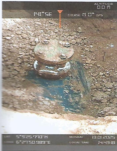
Fig 1. Showing the incident point after excavation.
